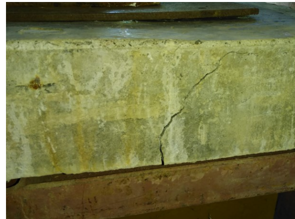
Fig 9: Appearance of crack near support
